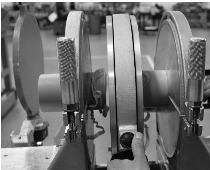
Figure F-13. The spigots of the fittings have to be planed with a planing tool. Ensure that the spigots of the fittings are always planed before every weld.
