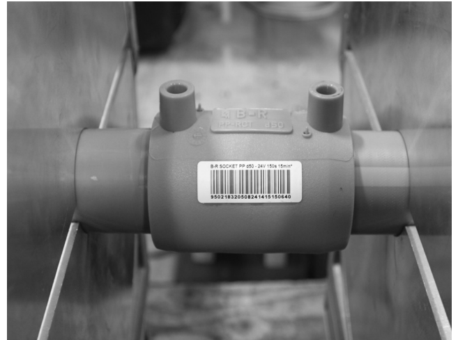
Figure F-19. Align the pipes and the electrofusion socket by using an aligning tool.
