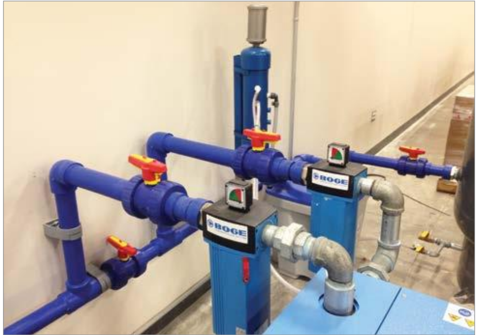
Asahi/America's Air-Pro ® specially formulated PE piping system installed at a manufacturing facility.
