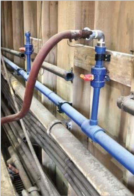
Asahi/America's Air-Pro ® , covered in chemical dust, safely operating at a fertilizer manufacturer.
