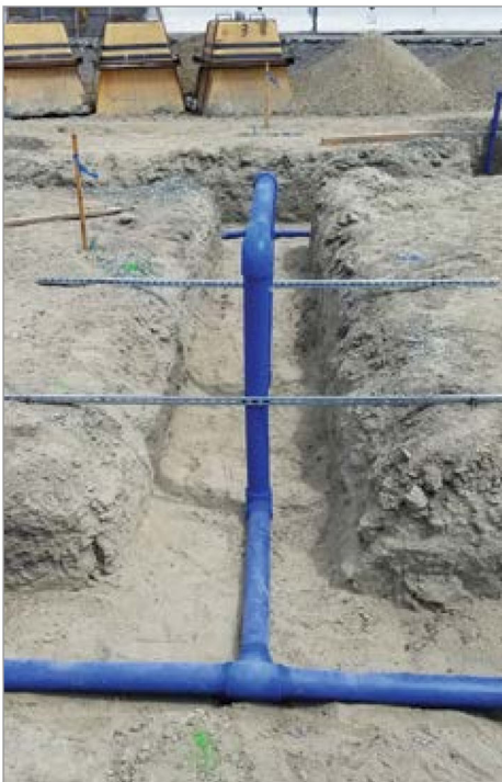
Asahi/America's Air-Pro ® in a buried application at a railroad station.
