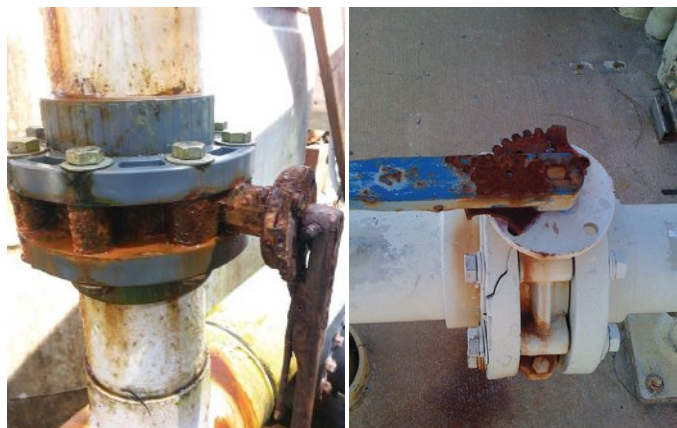
Rust is a common problem facing metal valves that thermoplastics are able to sidestep.
